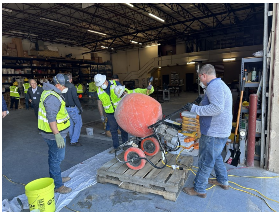
Participants mix concrete repair material under the watchful eye of Ben Koehler.
